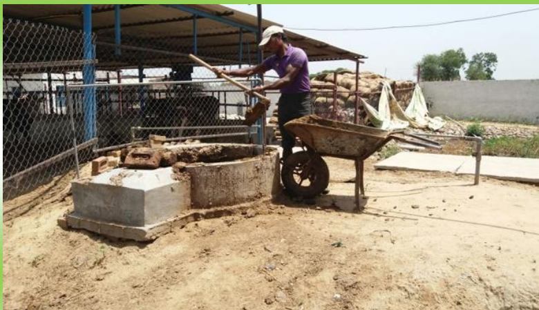
A labourer at work at a biogas plant at Loharan village in Jalandhar. (HT Photo)
