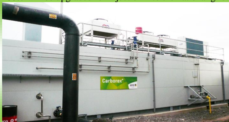
The new AD plant will supply up to 25% of the First Milk creamery's energy requirements
